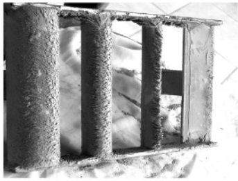
图 6 高温过热器区采样管结渣 Fig. 6 Slagging in the sampling tube in the high temperature superheater zone
