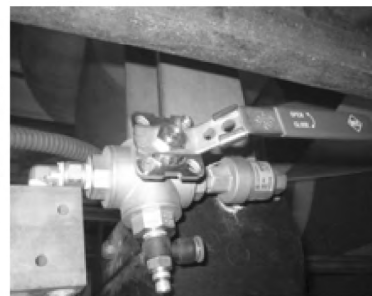
图1 抽汽逆止阀门手动操作活动试验装置 Fig. 1 Steam extraction non-return valve manual operation flexibility test device
